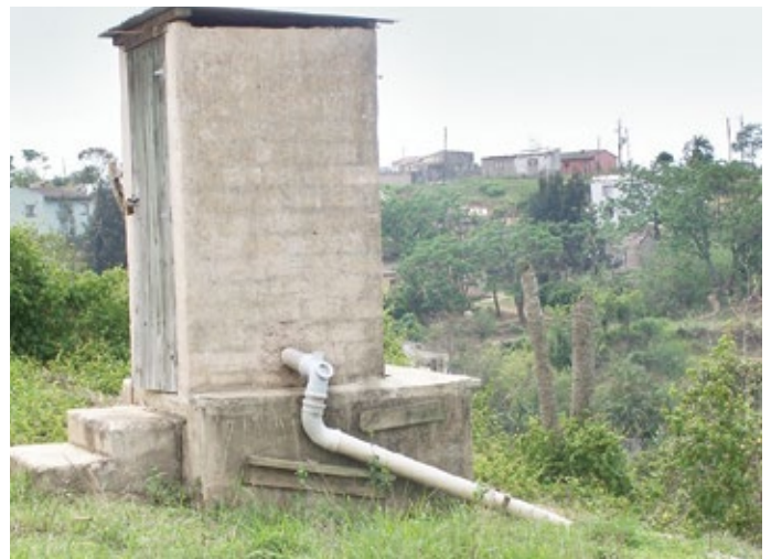
Figure 1: Some users converted their urine-diverting toilet to a flush toilet.
