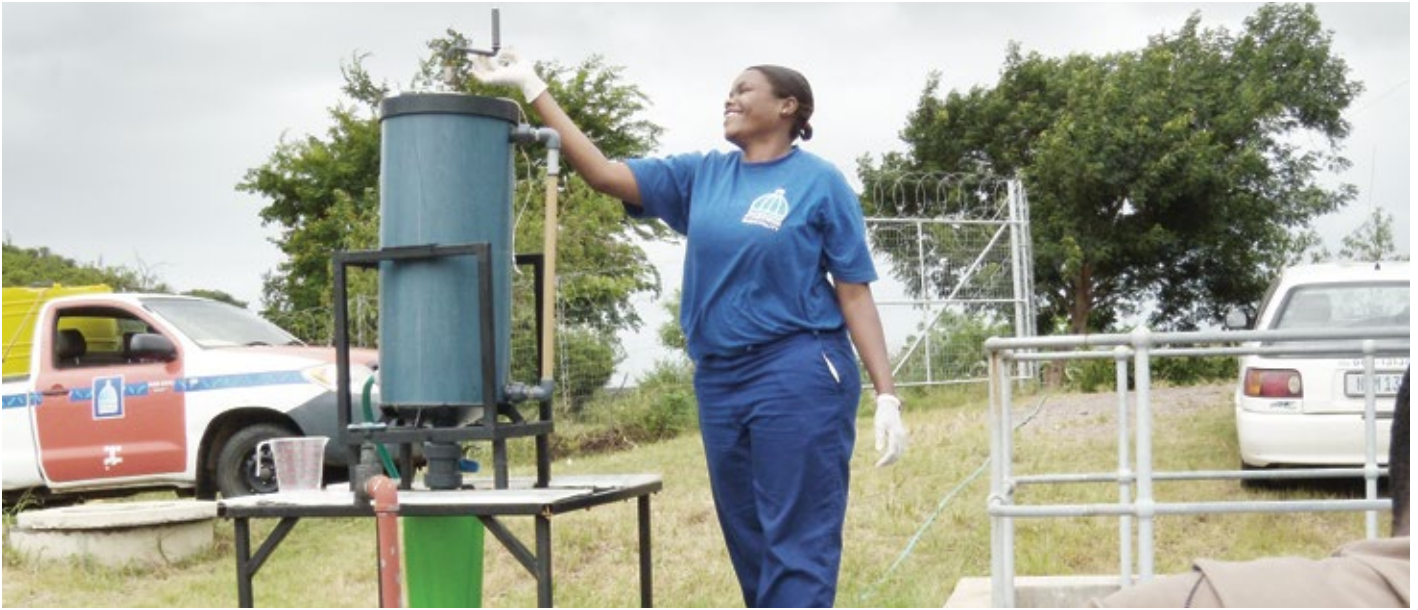
A manually operated struvite precipitation plant at the Newlands-Mashu Field Test Site.
