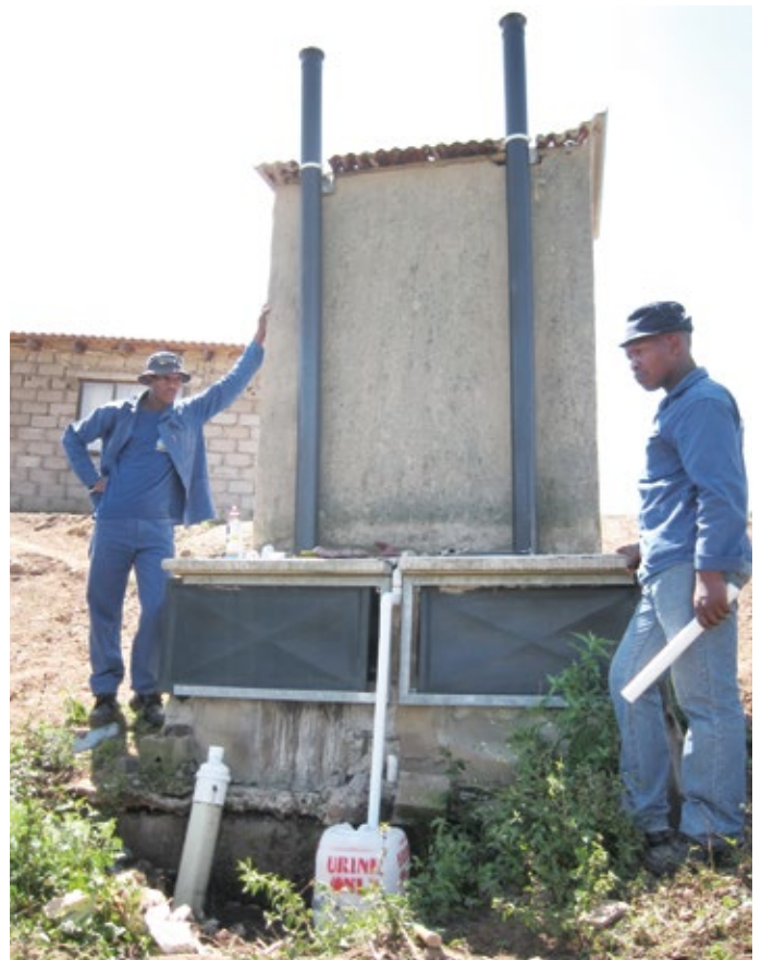
Figure 1: Municipal workers connect a 20-litre urine tank to the urine-separation pipe at a household toilet in eThekweni.
