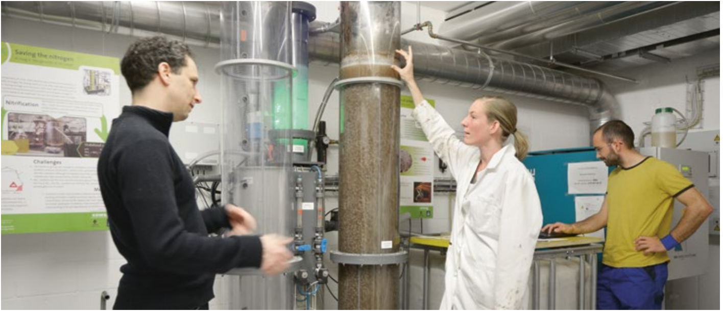
The nitrification and distillation plant in Eawag's basement is one of three pilot plants producing liquid fertiliser from urine.
