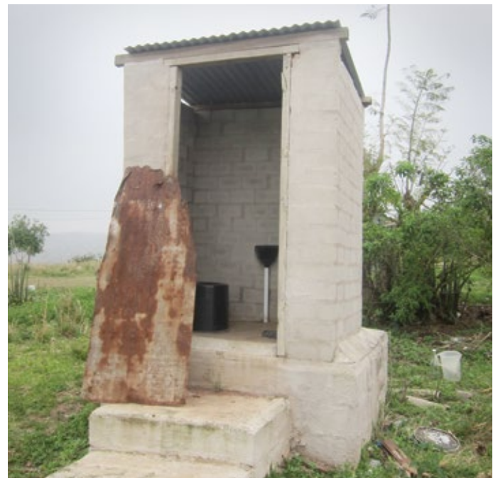
Figure 4: Some users were not satisfied with their urine-diverting toilet, because the doors were stolen or damaged, or the vent pipes were dysfunctional.
